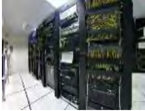
Data Center Infrastructure
